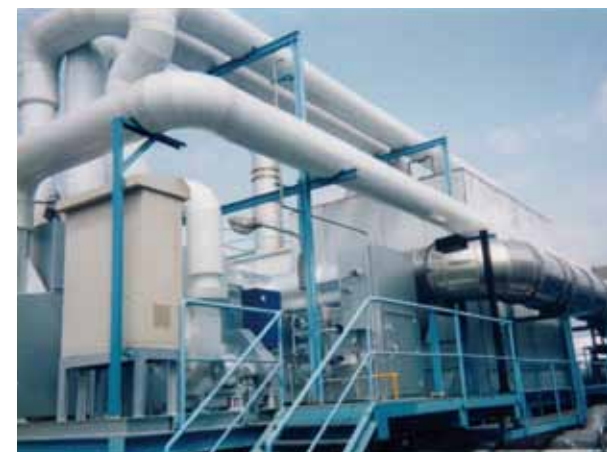
VOC abatement system including thermal oxidizer & concentration cassette
